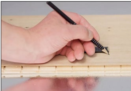
The last plank of the first row is shortened to the required length, taking into account the wall clearance. The cut-off piece of the plank is used as the start of the second row.
