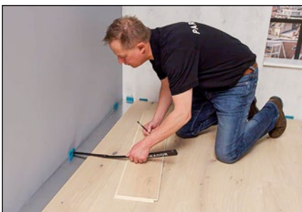
Use a leftover piece or the Parador MultiTool to transfer the wall outline to the last row of planks.
